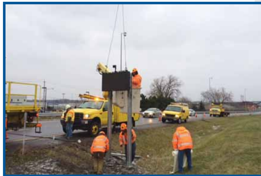
New York State Thruway employees install a Wrong Way Deterrent Sign system at the Thruway's Buffalo exit in December 2013. Commenting on the installation in Buffalo, Governor Andrew Cuomo said, "New York is the first state in the nation to utilize this sophisticated technology to enhance traffic safety and save lives."
